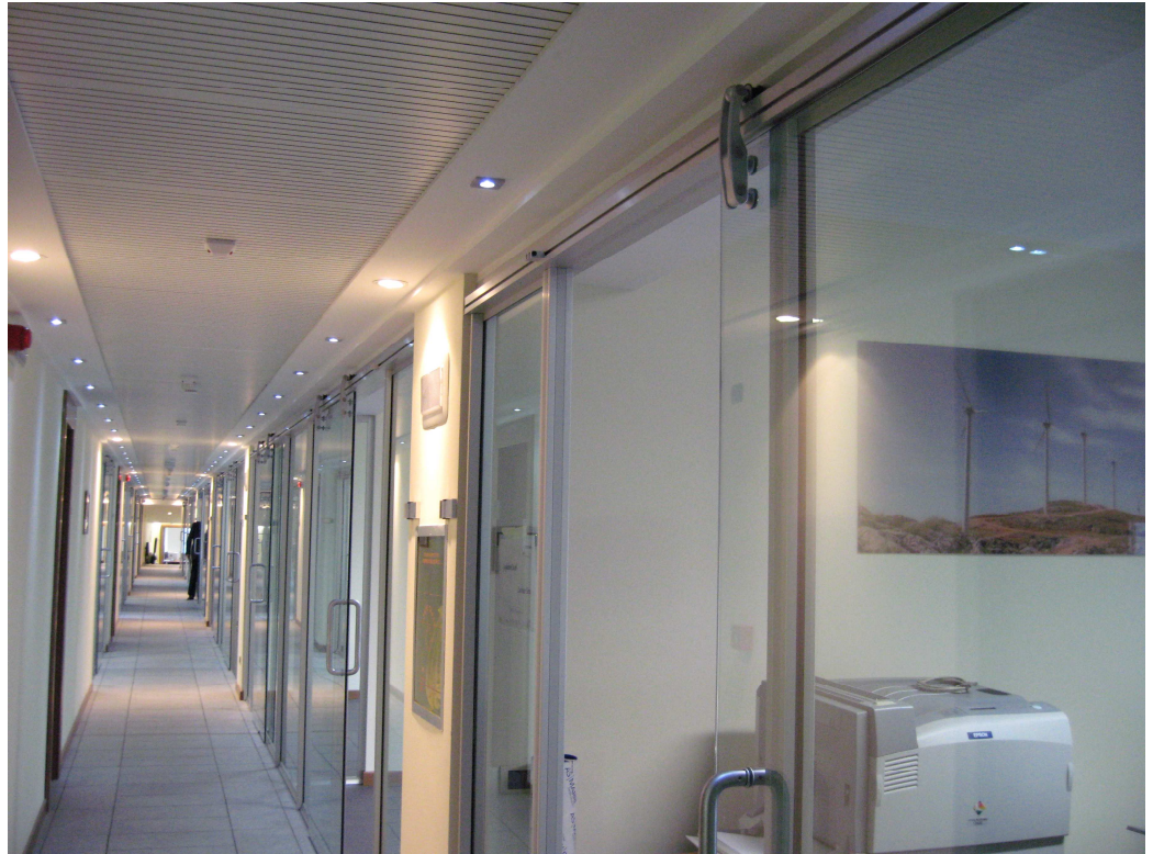
The corridor in the section along Via Bordonni, where a false ceiling was made in slatted MDF, with inserted LED spotlights, totally serviceable porcelain floating floors and glass walls with sliding doors
