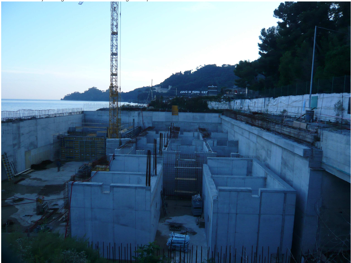
The Santa Margherita wastewater management plant under construction; the drive-in tunnel entrance can be seen in the foreground to the right
